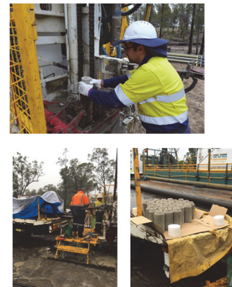
Fig 3: 467 bentonite plugs were placed successfully on top of the grout to reach final top of plug at 6m GL as per program.
