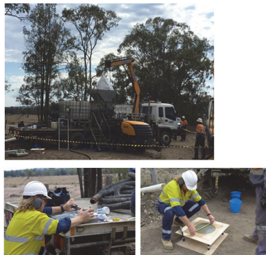
Fig 2: 205l of 1.94SG grout was mixed and pumped in hole. After 3h WOC the top of grout was tagged at 94.7m GL.
