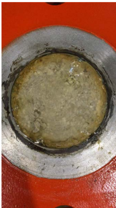
Figure 29: 5A-PVP in a 4" pipe/ third hydraulic test. Air bubbles occur at the interface plug/steel pipe at failure pressure.
